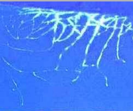
Cracks clearly visible after fluorescent spray
